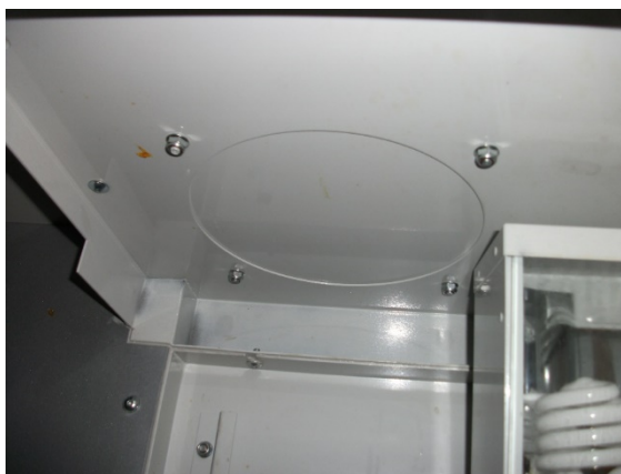
Figure 5.3 Interface for LEV as seen from inside a CNC enclosure.
